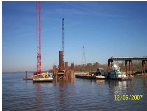
The work trestles, when complete, will allow crews to work on the main span bridge regardless of the river conditions.
