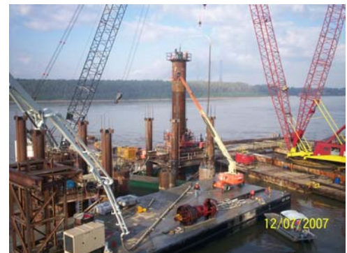
Crews work in the Mississippi River on the main span bridge shafts
